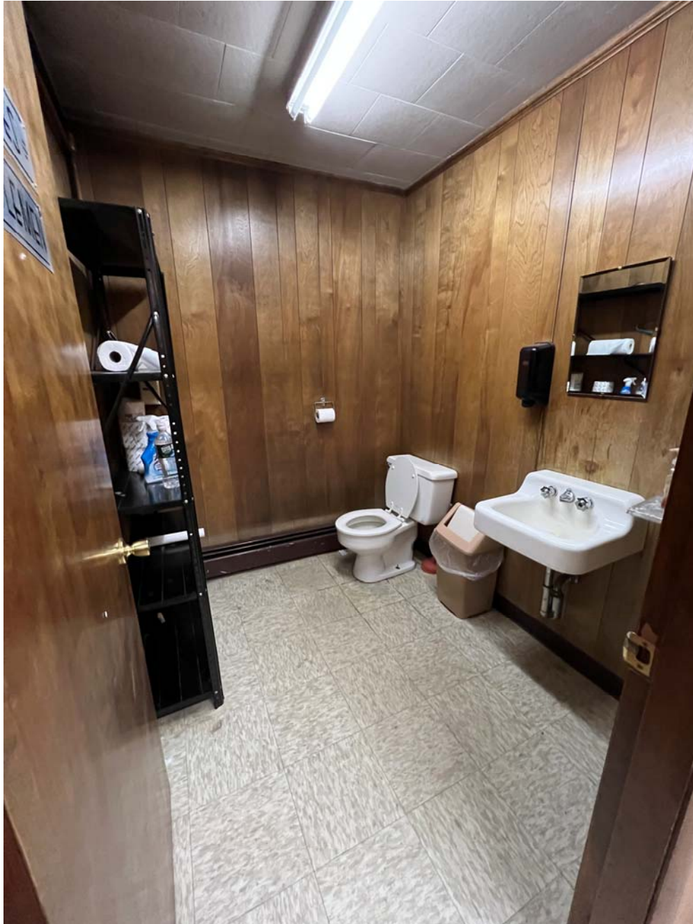
Existing Bathroom needs upgrades
